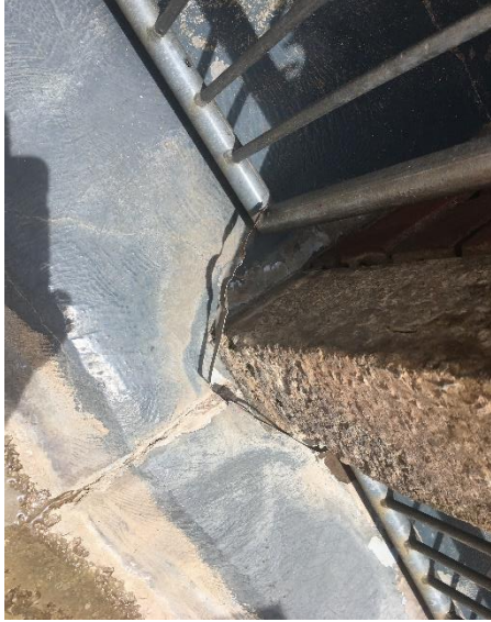
Figure 5: shows the sharp protruding wires.
