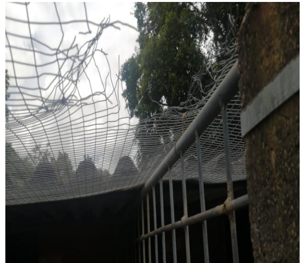
Figure 24: shows the hole in the fencing.
