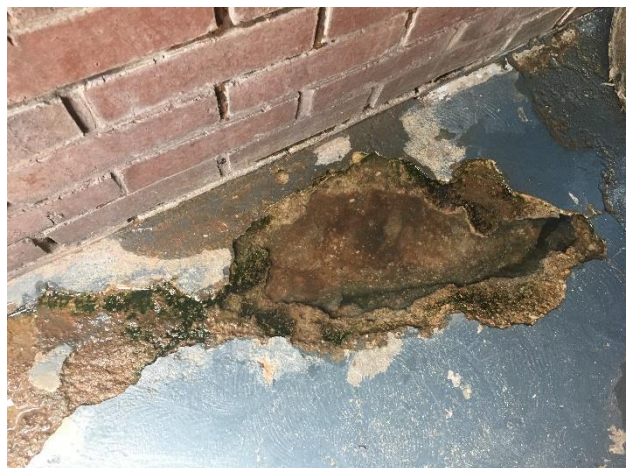
Figure 4: Shows the holes in the flooring in one of the kennels.
