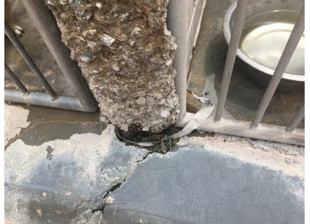
Figure 22: Shows the protruding wire brackets.
