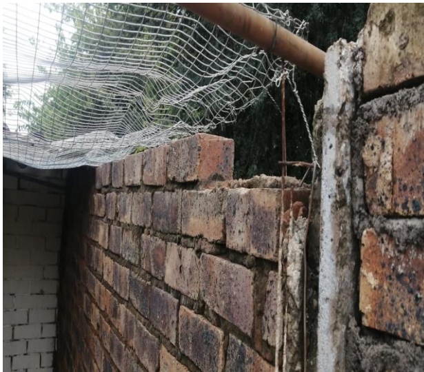
Figure 23: Shows the hole in the fencing.
