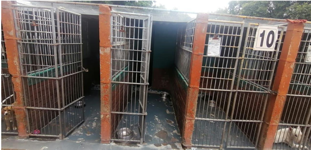
Figure 10: Shows the dilapidated state of the kennels.
