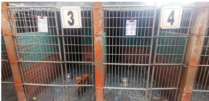
Figure 9: Shows the dilapidated state of the kennels.
