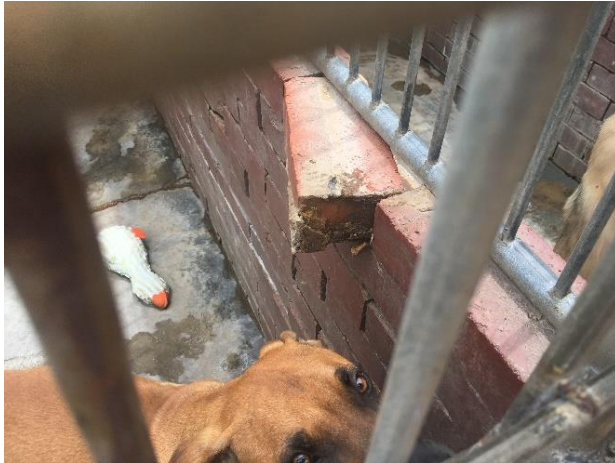
Figure 21: Shows the loose brick in one of the kennels.
