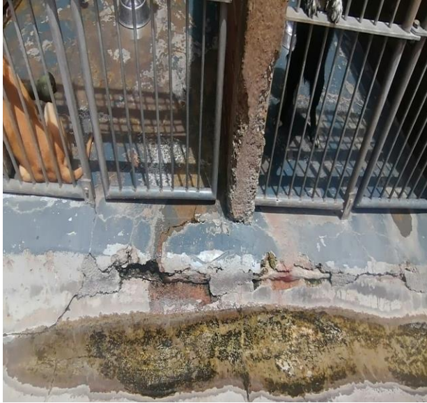
Figure 14: Shows the dilapidated state of the kennels and the algae in the drains.
