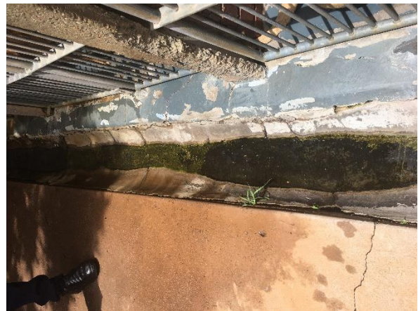
Figure 8: Shows the algae build up in the drainage system.
