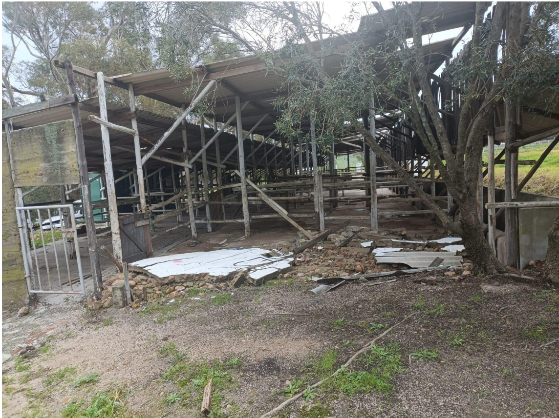
Photo 16: Delapidated shelter destroyed by storm.
