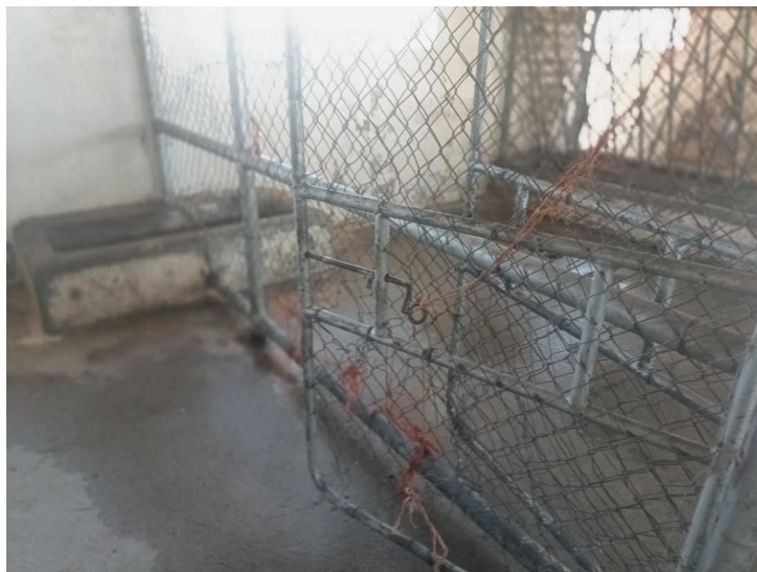
Figure 4: Broken fencing in calf indoor night shelter.
