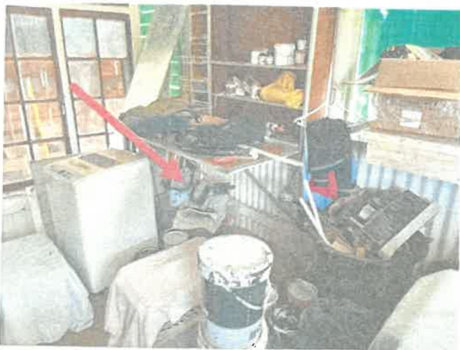
Photo 1: Open paint container (red arrow) amongst the other debris.
