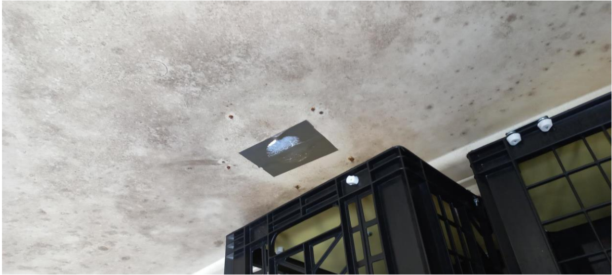
*Sealed ventilation hole 2 in front section. To be reopened and turned into a proper ventilation hole.
