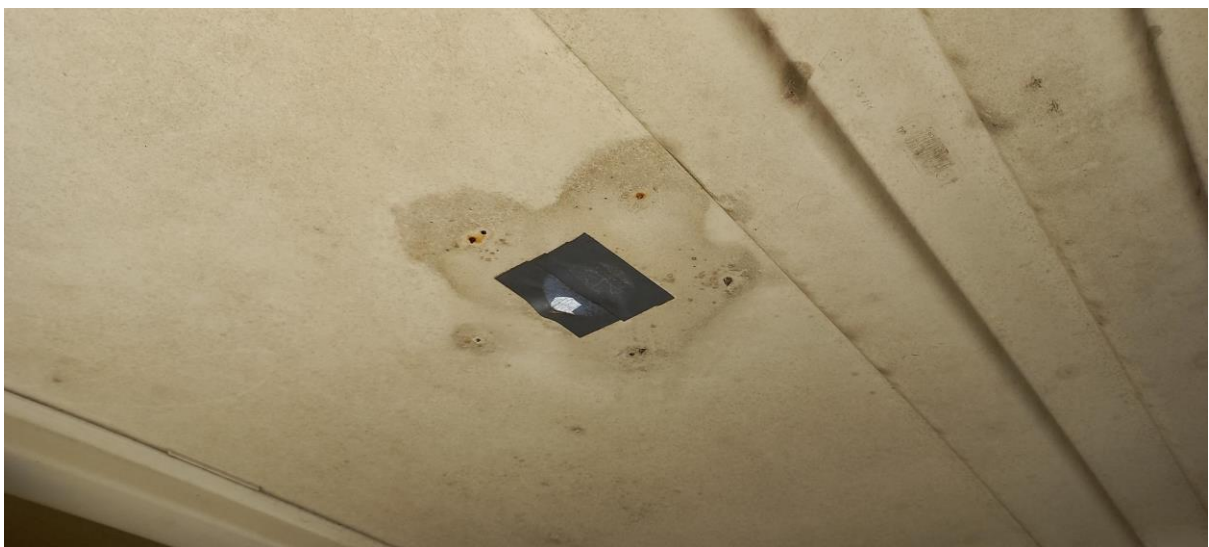
*Sealed ventilation hole 1 in front section. To be reopened and turned into a proper ventilation hole.
